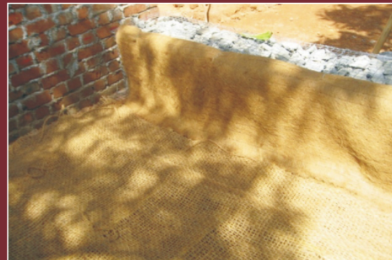
Fig. 7. Laying of woven coir geotextile as reinforcement and non-woven coir geotextile as filter
