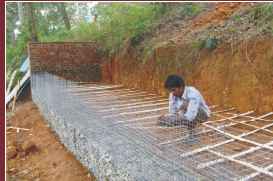
Fig. 6. Placing of gabion boxes and laying of bamboo reapers for the second layer of retaining wall.
