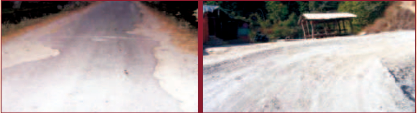
FIGURE 5. Edge breaking and raveling on curves.
