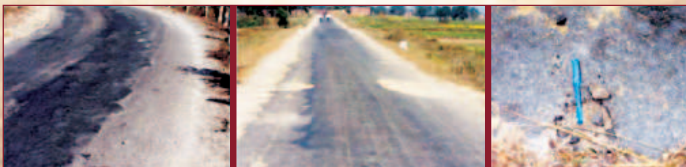
FIGURE 4. Rutting, potholes and scaling.
