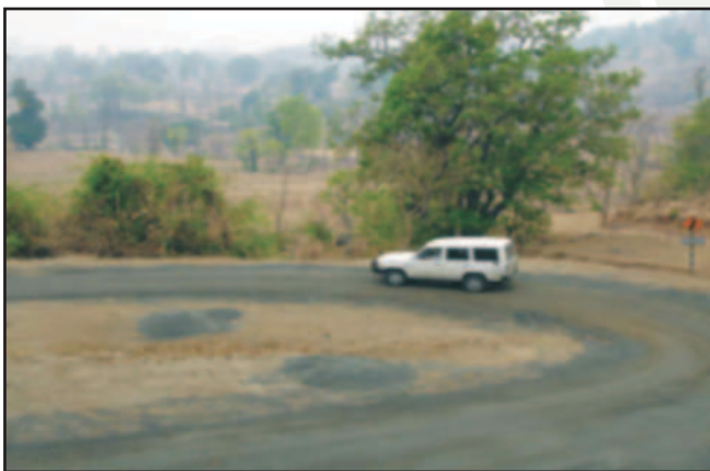
Photograph 4 - Road Safety Hazards due to Sharp Curves on PMGSY Road
