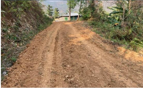
Existing Damaged Road
