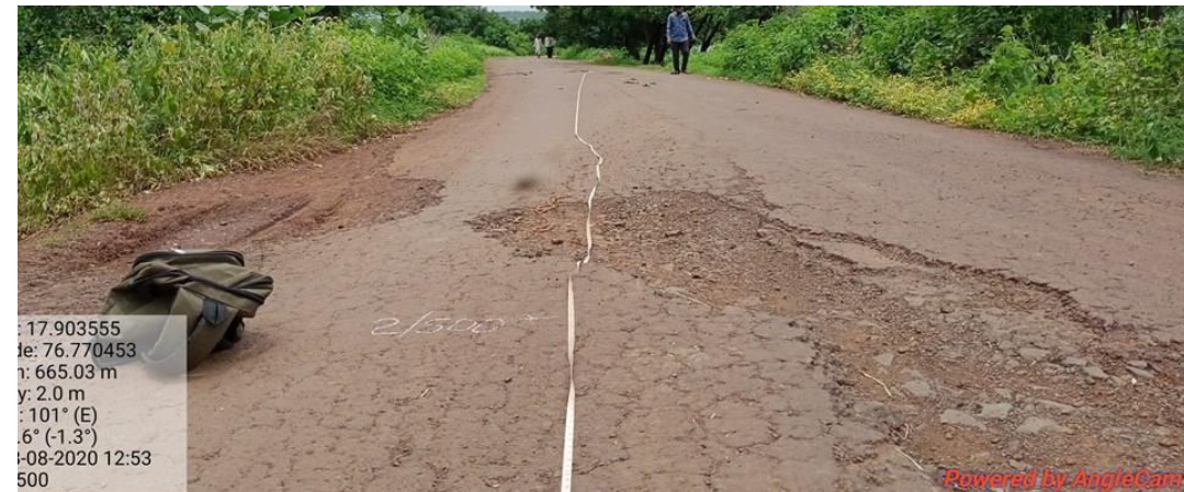
Potholes and Cracking
