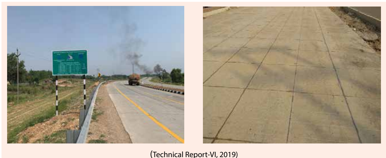
Figure 2: A view of Short Panel concrete pavement (SPCP) on NH-18 (old NH-33) (Year 2017)
