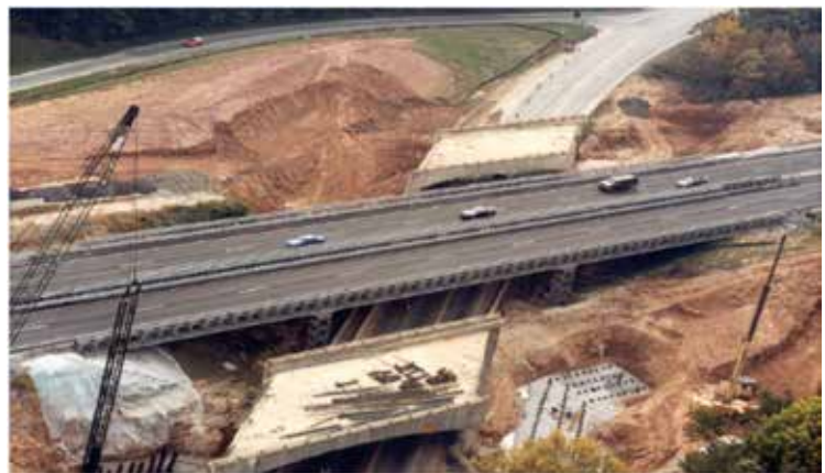
Figure1: Temporary Modular Bridge in service while construction of permanent bridge in progress
