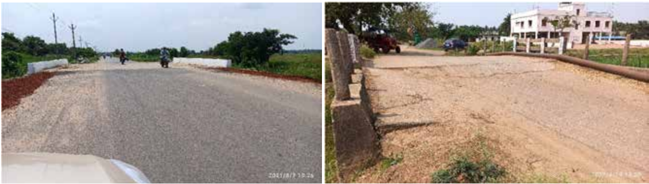
Figure 1: Bridge approach failure with the formation of a bump
