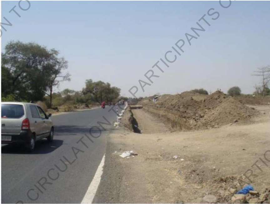
Unprotected foundation trench in work zone
