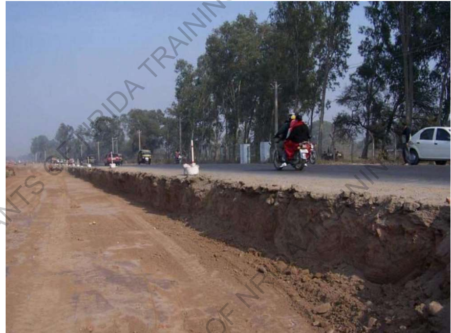
Unprotected vertical cut close to traffic
