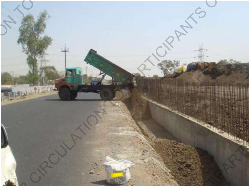
Unsafe operations in work zone
