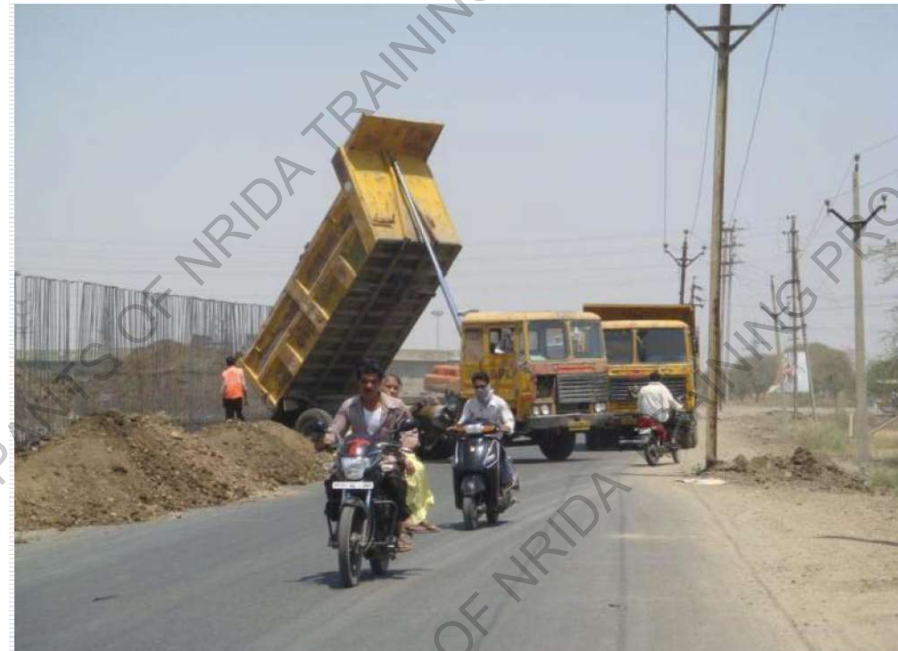
Absence of demarcation and buffer zones in work zone
