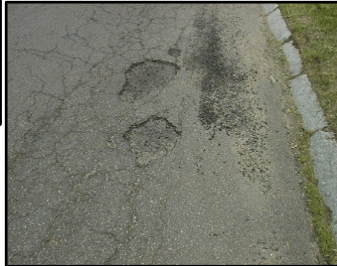
Moisture induced damage
