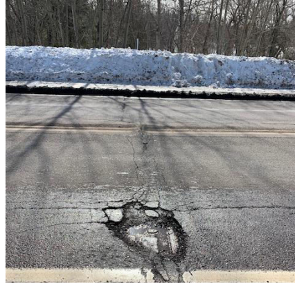
Pothole (moisture damage)
