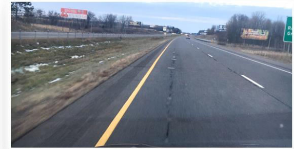
Top-down Fatigue Cracking
