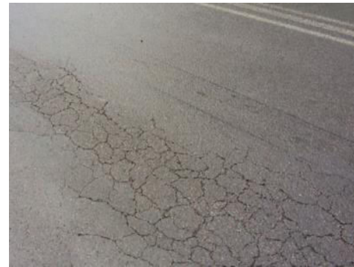
Bottom-up Fatigue Cracking
