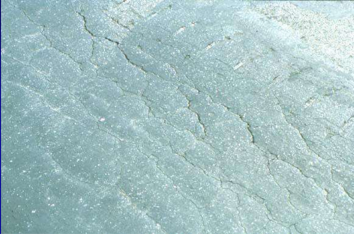
Fatigue Cracking and Rutting
