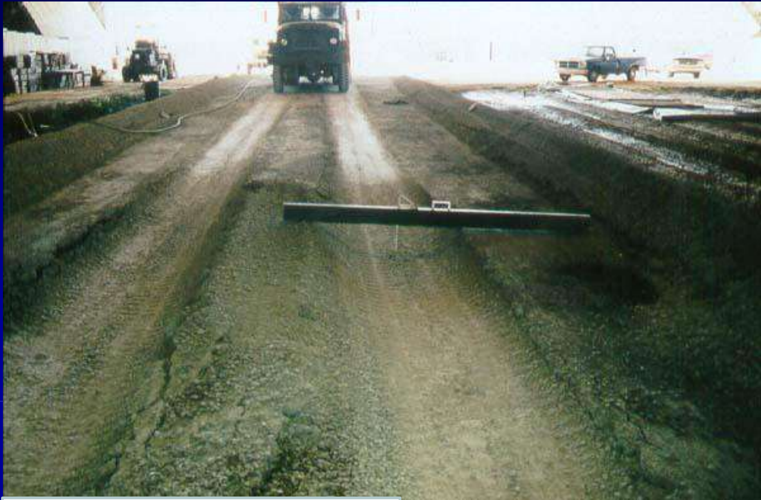
Rutted Section of Unreinforced Road
