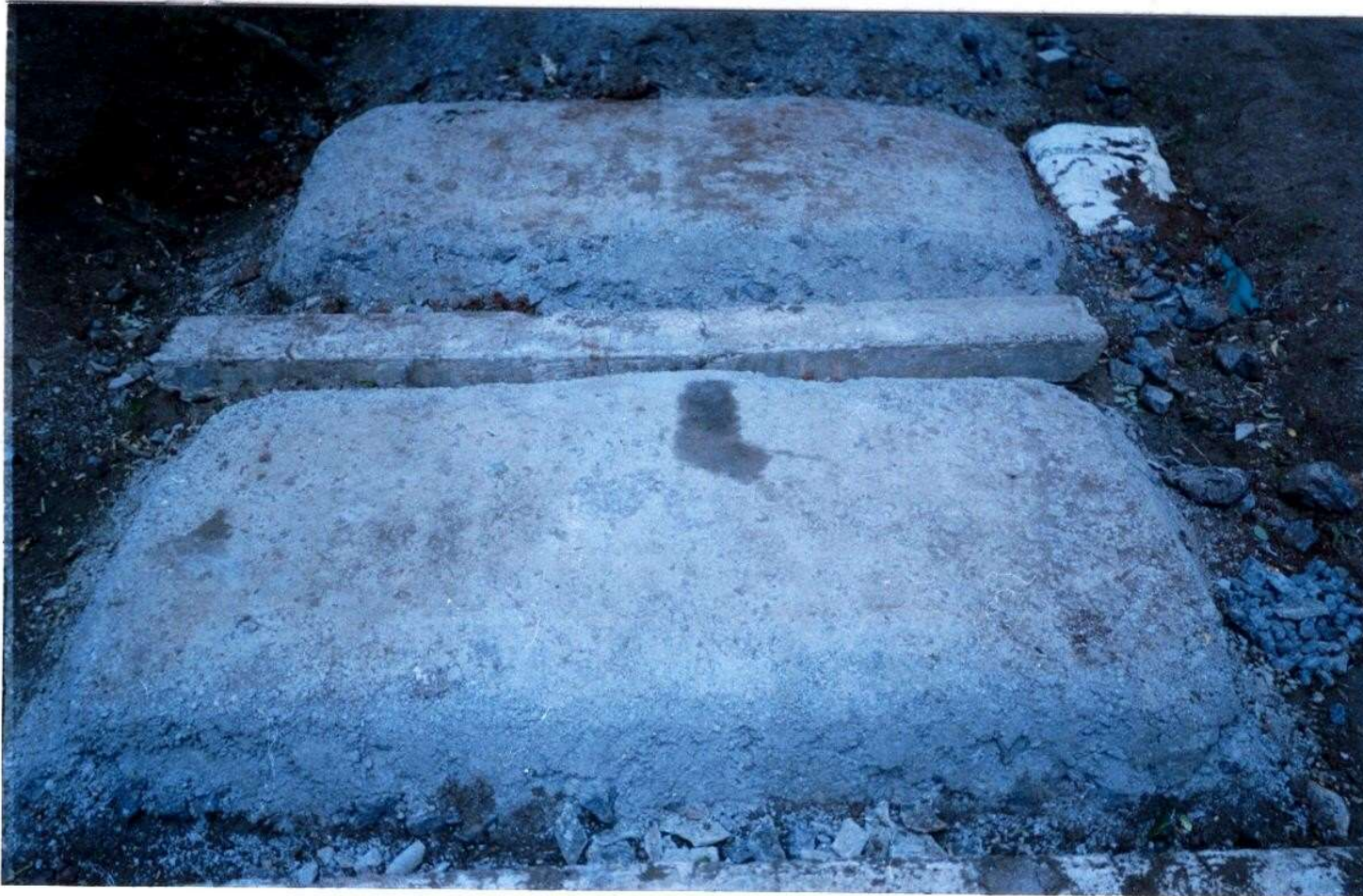
Plate 4.3 Cement stabilized WBM stretch after monsoon rains
