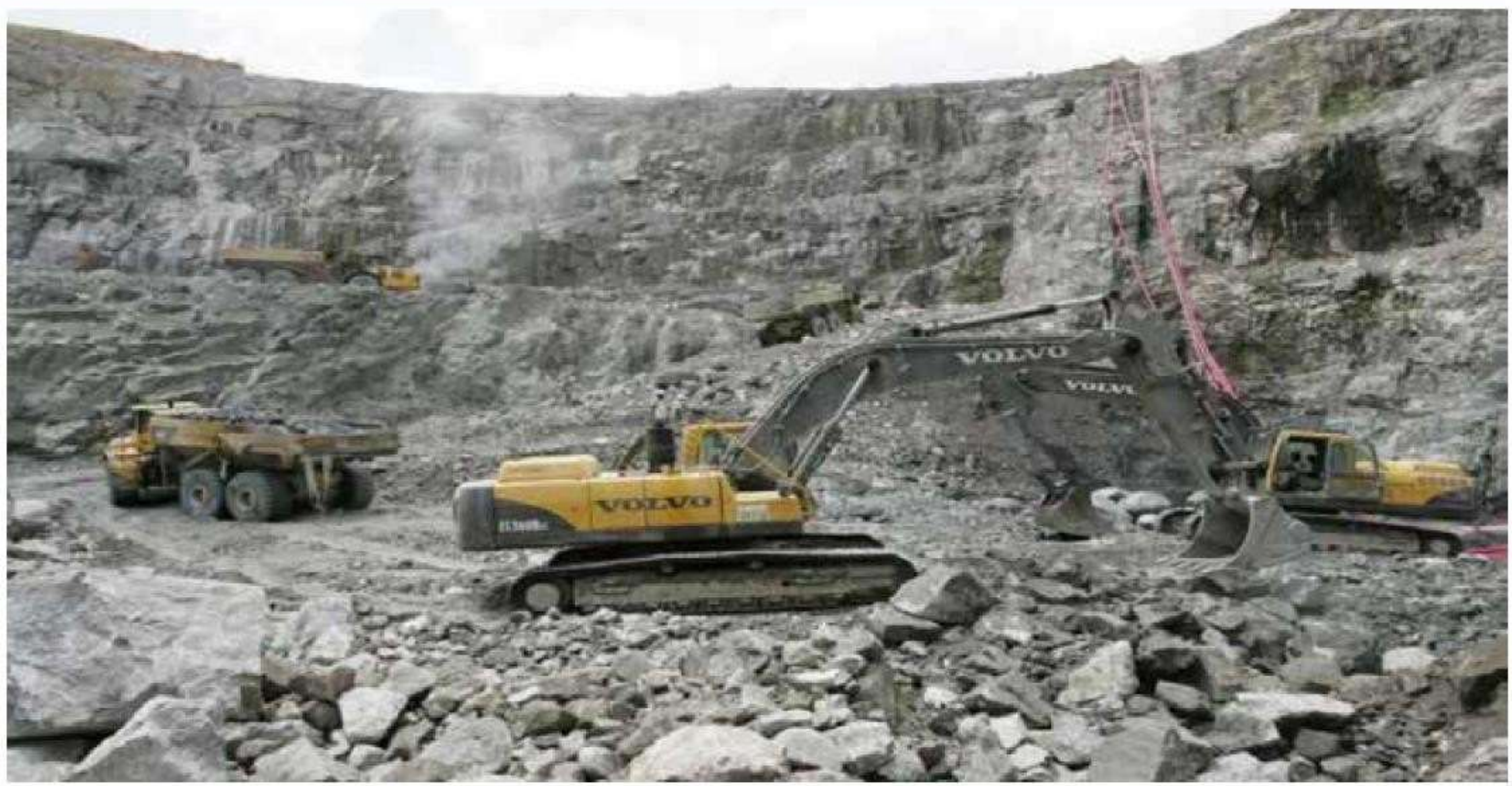
FIGURE 1: Destroying our valuable mountains for the quarrying of aggregate
