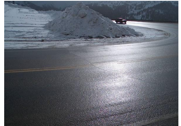
➤ Low temperature cracking
