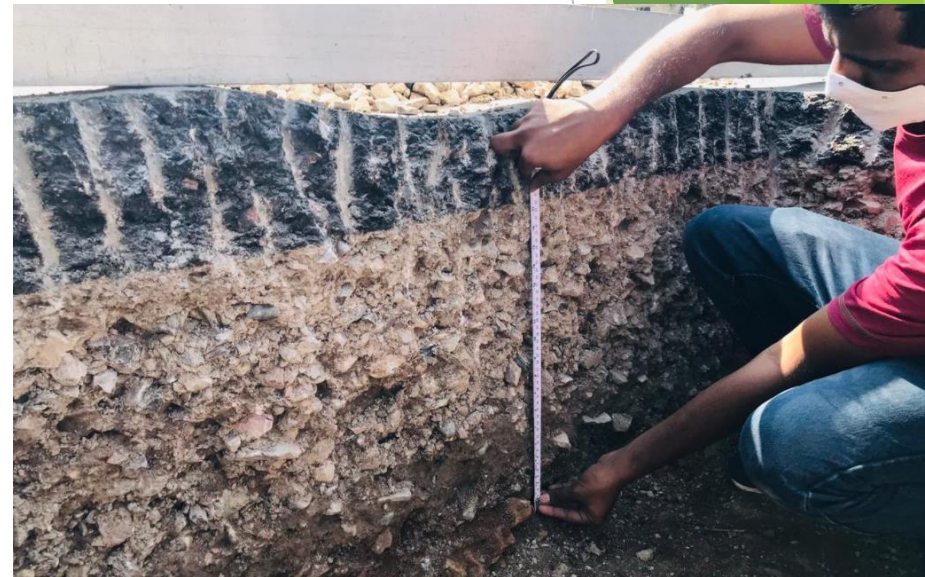
A test pit taken in a high volume road exhibiting rutting
