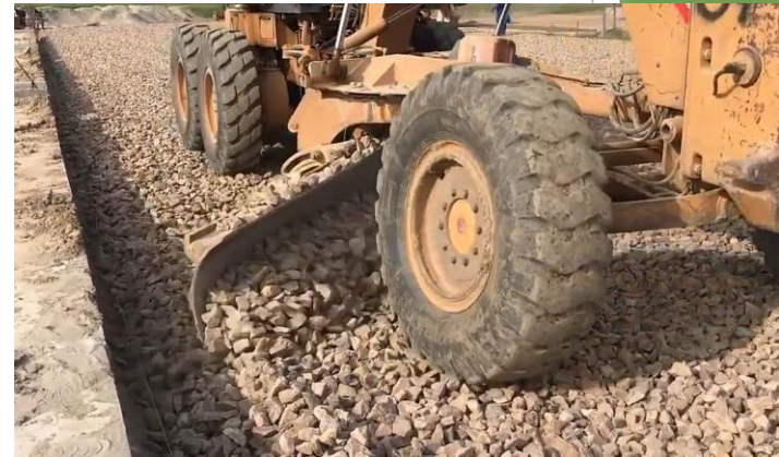
Ensuring that sufficient loose qty of material is spread - checking with string lines
