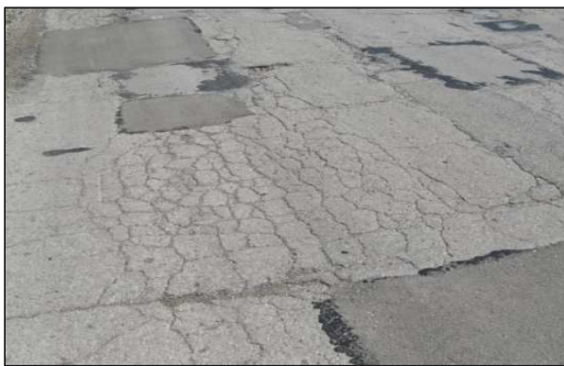
Fig 4.19: Depression and resulting cracks
