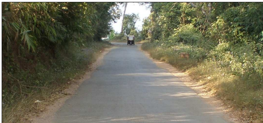
Fig 3.6: Rural road in need of off-carriageway routine maintenance
