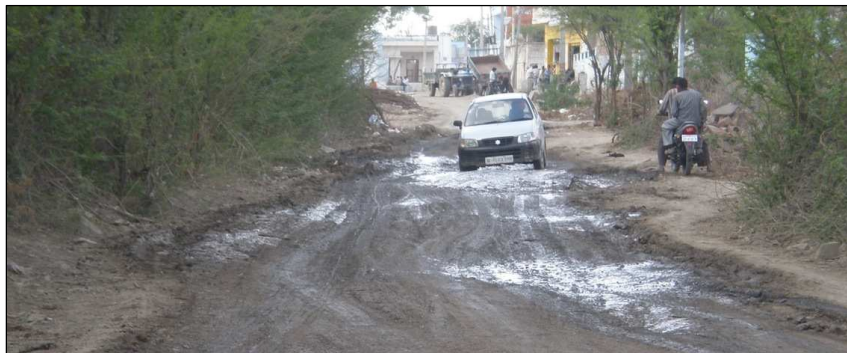
Fig 2.4: Rural road deteriorated to the extent that full rehabilitation is required.
