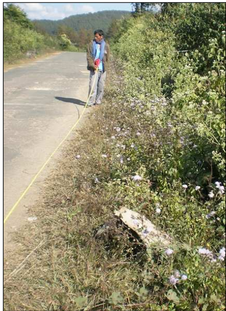
Fig 4.10: Need to clear bush in side drains
