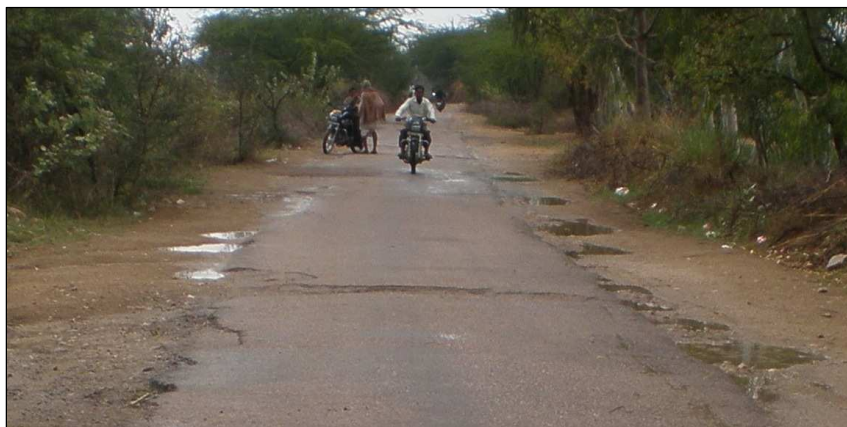
Fig 4.20: Stagnant water on shoulders
