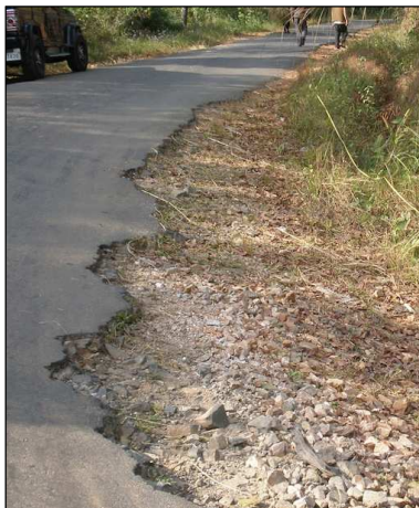
Fig 4.14: Edge of pavement breaking
