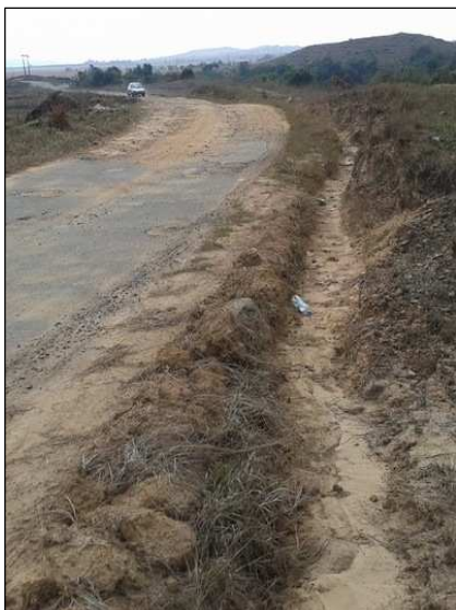
Fig 4.7: Silt accumulating in side drain
