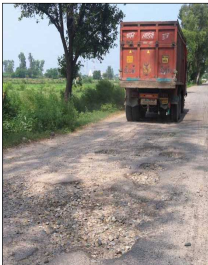
Fig 1.3: Lack of maintenance causing higher vehicle operating costs and increasing costs of transport services
