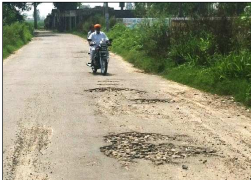
Fig 4.13: Poor quality aggregate in base course causing premature potholes
