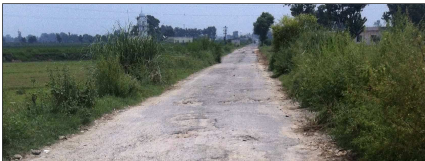
Fig 4.6: The lack of maintenance of road shoulders has resulted in poor drainage of the surface leading to premature failure of the surface seal.
