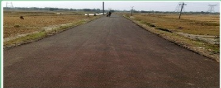
BitChem Coldmix Road at Jalpaiguri, North Bengal
