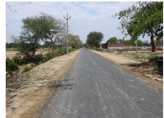
Condition of Road after 3 years
