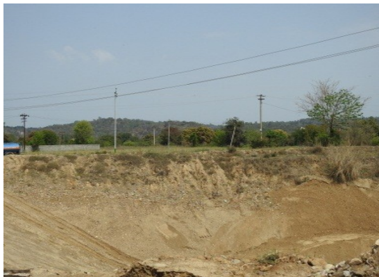
Eroded Slope of Cuttings
