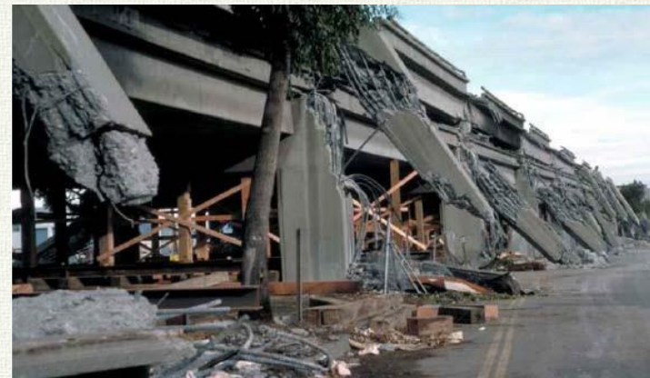
Weld failure of column longitudinal reinforcement: 1995 Kobe Earthquake.
