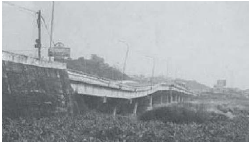
Failure of Bridge deck slab
