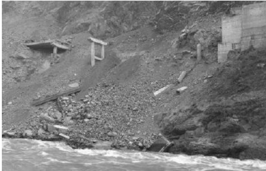
Yiwanshui Bridge Collapse by stone hitting
