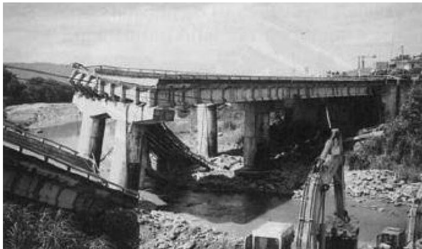
Failure of Shiwei Bridge
