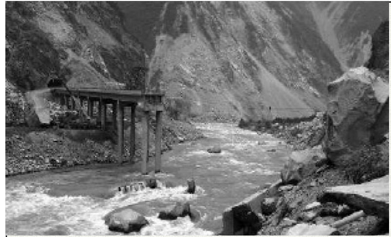
Chediguan Bridge 1-3 Span Collapse by stone hitting
