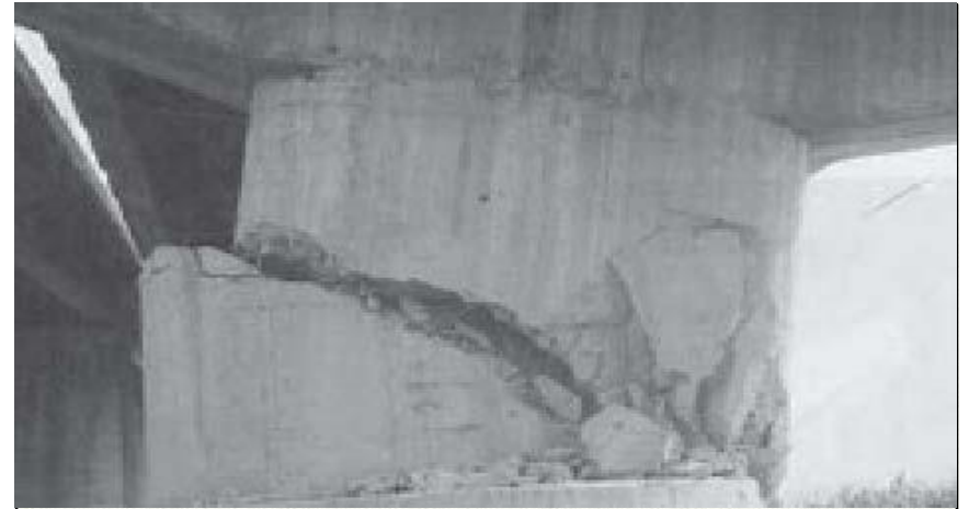
Shear Failure of Bridge pier
