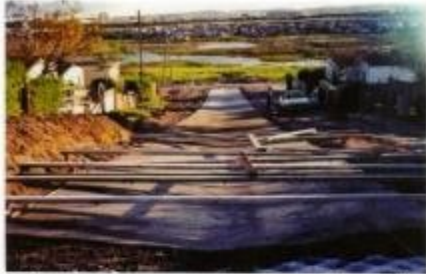
Road and drain incorporated. Drain can also be to side of road. (Hall & Hall 2007).
